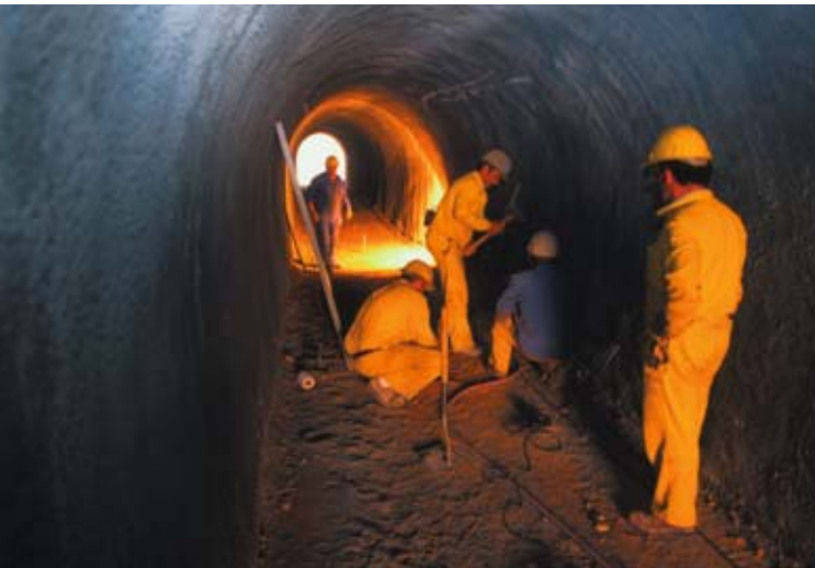
A drinking water conveyance tunnel in Valencia (Spain).
