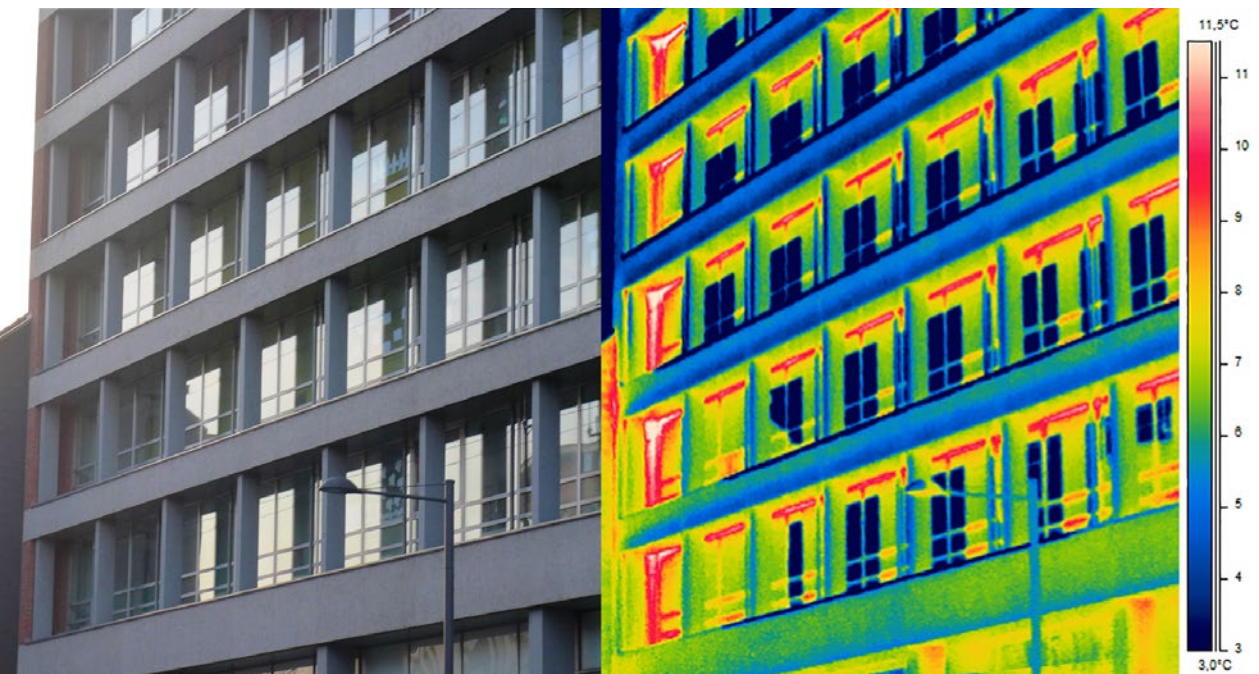
Thermal image of the facade of the crèche building showing heating loss (energy audit began in March 2017)
