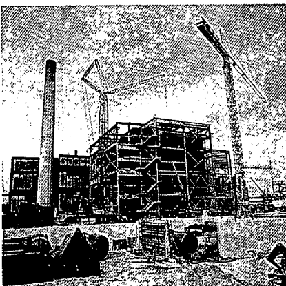
Coal heating plant, Saint-Ouen
