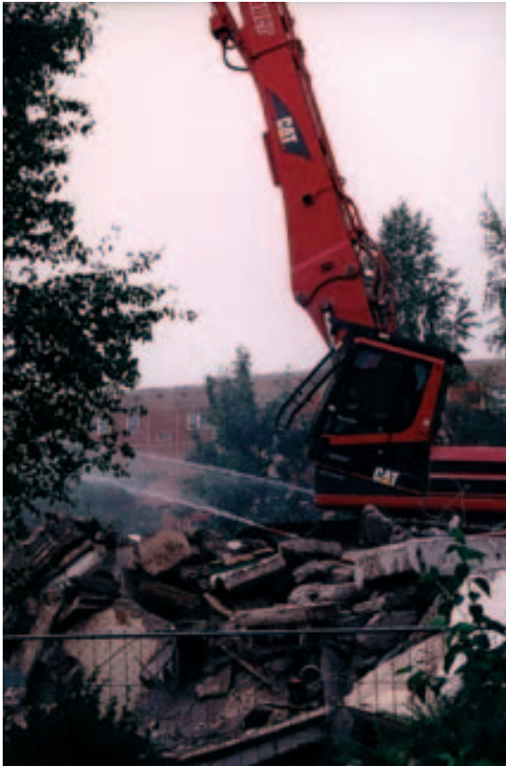
Watering of the working area to reduce the emission of dust and fibres
