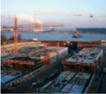
Prefabrication of two tunnel elements in the dock beside the river (courtesy of Heinrich Hirdes GmbH)
